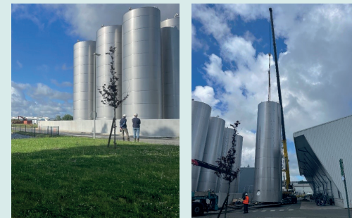
Expansion of our tank farm
